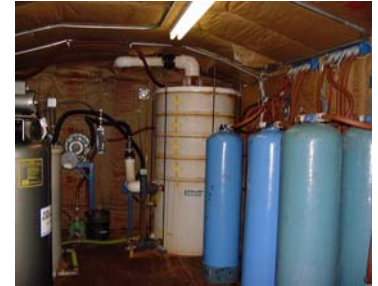
Air stripper (background) and granular activated carbon canisters (foreground) for removing MTBE.
