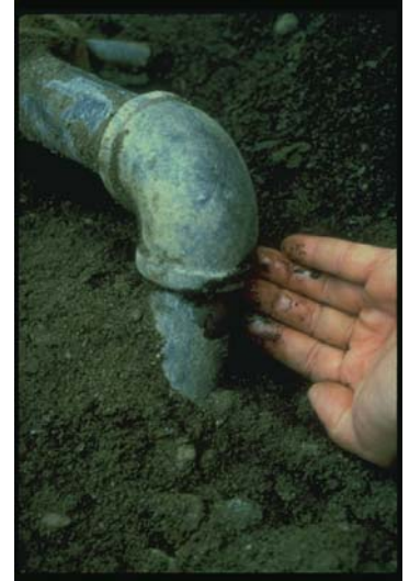
Leaking Product Line
