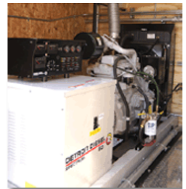
Diesel generator for MMPE unit
